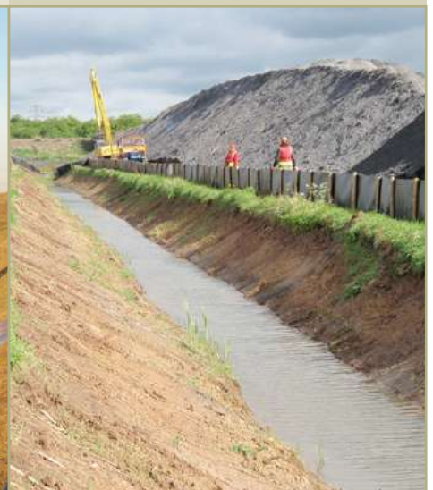
Installation of water vole fencing using our offset trencher Photos: Legacy Habitat Management
